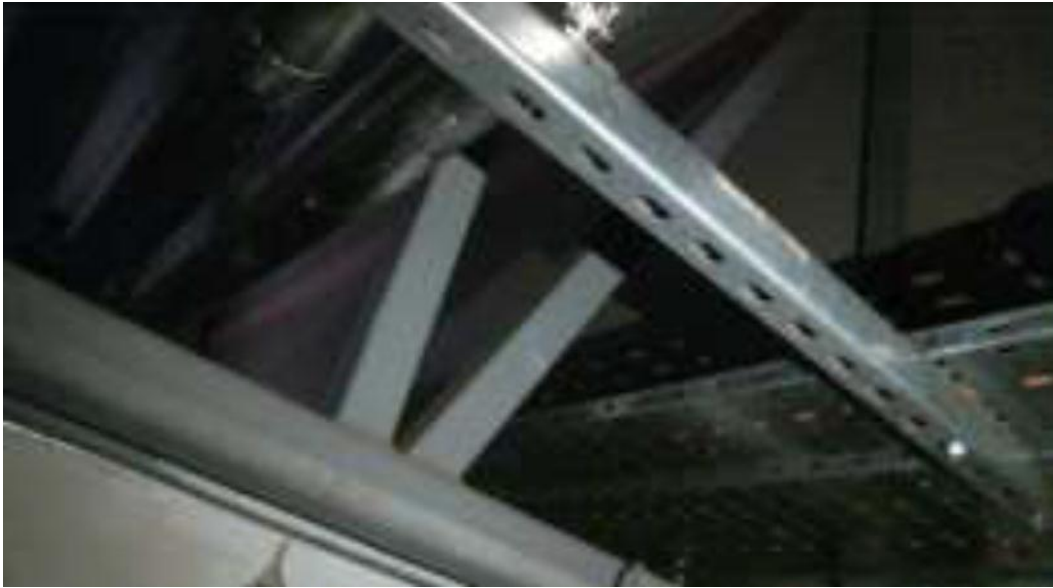
Image 21: Example of a breach of fire compartmentation from fire-stopping survey of Oxgangs School, dated 22 nd August 2016: "there is no plasterboard above the fire door, therefore creating a large breach in the compartment. the area is not fire stopped and a breach exists."
