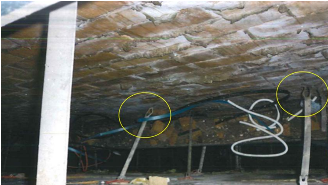
Image 28: Photograph from Duncanrig Secondary School. 'Note wall ties with no embedment in outer brick leaf of cavity wall'.
