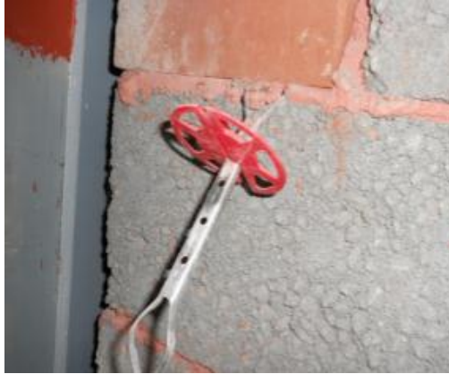
Image 29: St Ninian's High School; "Photo showing one of the defective wall ties (no embedment) in place behind the internal skin of blockwork in the sports hall."
